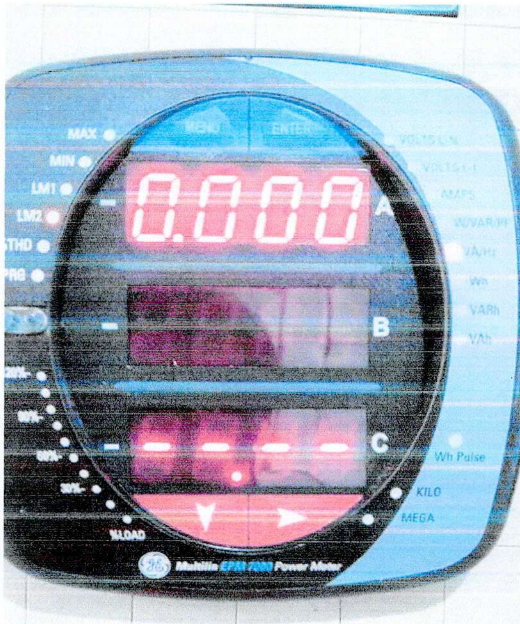
Item No. 10_Multimeter_Electro Industries Gauge Tech Shark 100
